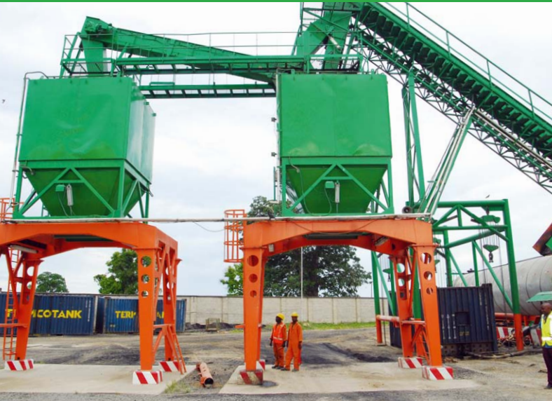
BAM International's own asphalt installation
