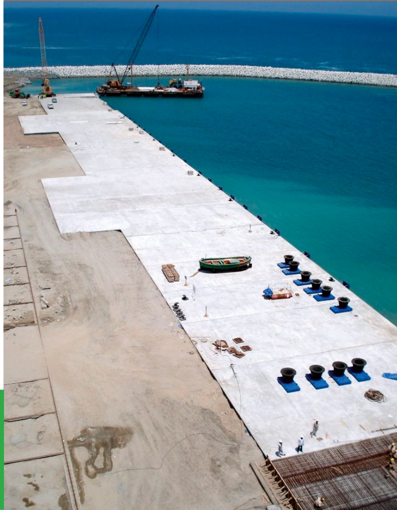
Finishing of the load out platform capable for loads up to 50 ton per m 2
